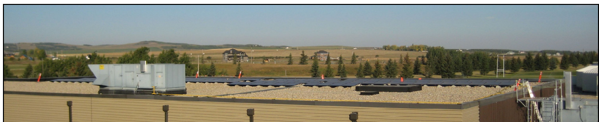
Figure 4 View of the complete installation looking from the East
