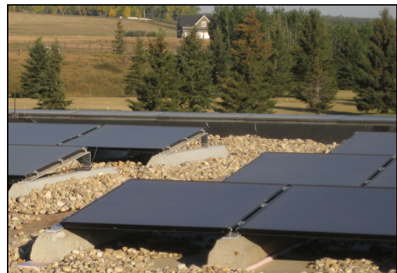
Figure 1 Close-up of the arrays and mounting structure
